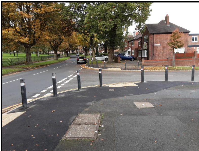
Firbank Road/Highdales Road, Baguley - Reconfigured junction/bollards/drop kerbs/tactile pavings/road markings/traffic signs/No Waiting at any time restrictions
